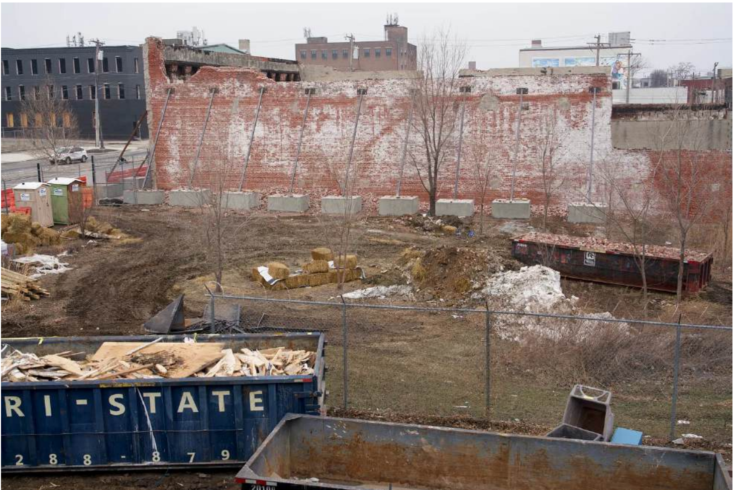
Image courtesy of Jon Kaufman of the construction site for Forman Arts Initiative.
